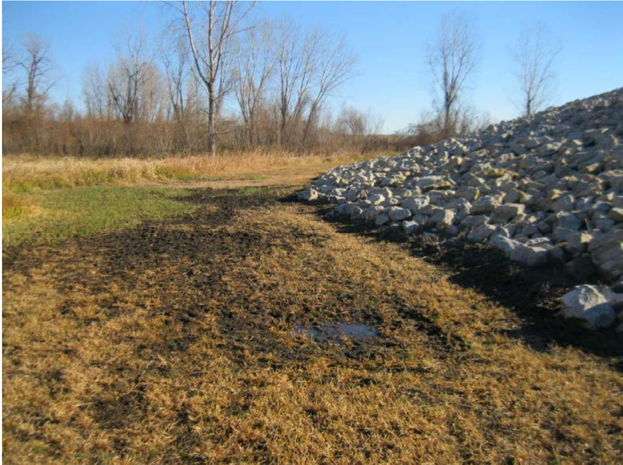
Figure 4-4 Standing Water along Toe of North Facing Slope
