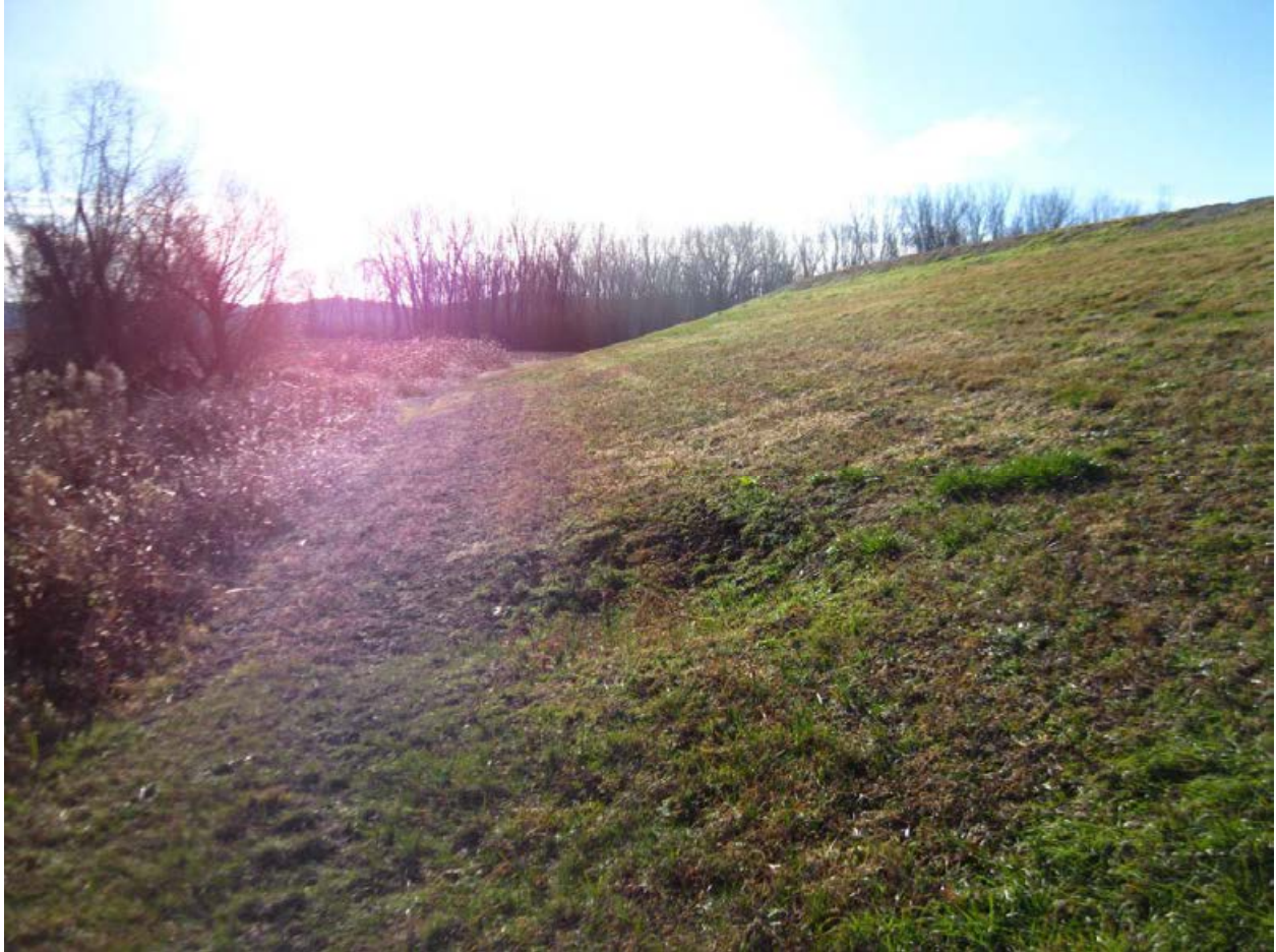
Figure 4-7 Minor Surface Irregularity Along East Facing Exterior Slope.
