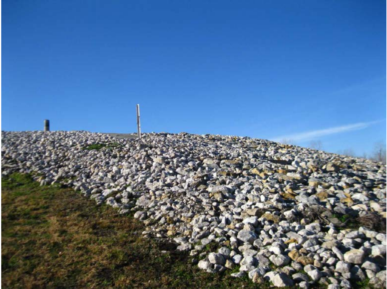
Figure 4-6 Exterior Dike Slope Surface East of the Plugged Discharge Pipe.
