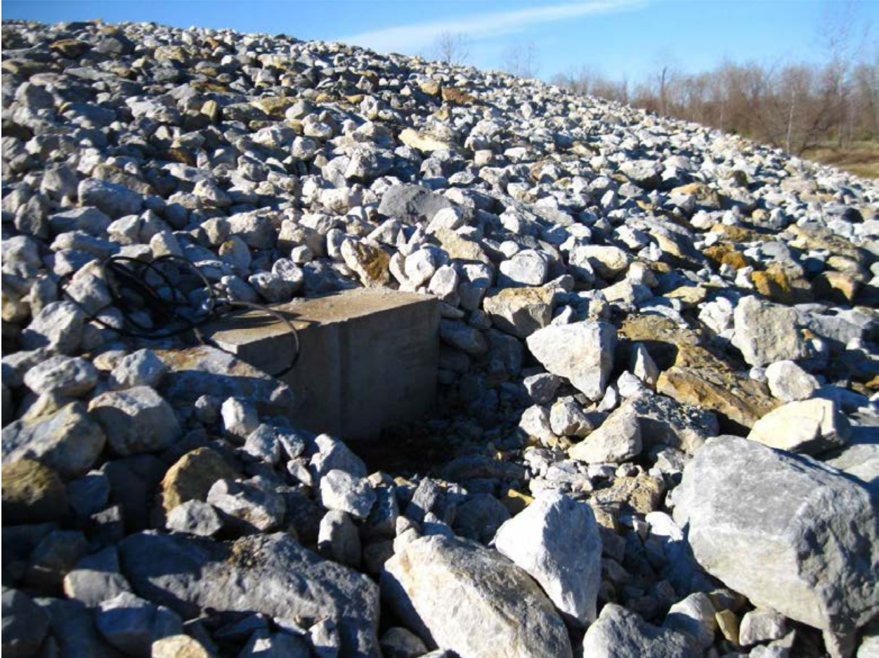
Figure 4-9 Bottom Ash Pond 30 Inch Diameter Plugged Discharge Pipe.
